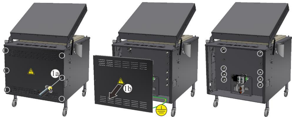
Fig. 75: Dismantle the cover of the switchgear from the back of the furnace (similar to picture)
